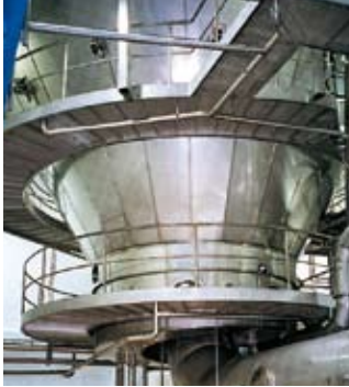
Conical part of spray drying chamber with the integrated fluid bed in a CDI Dryer
