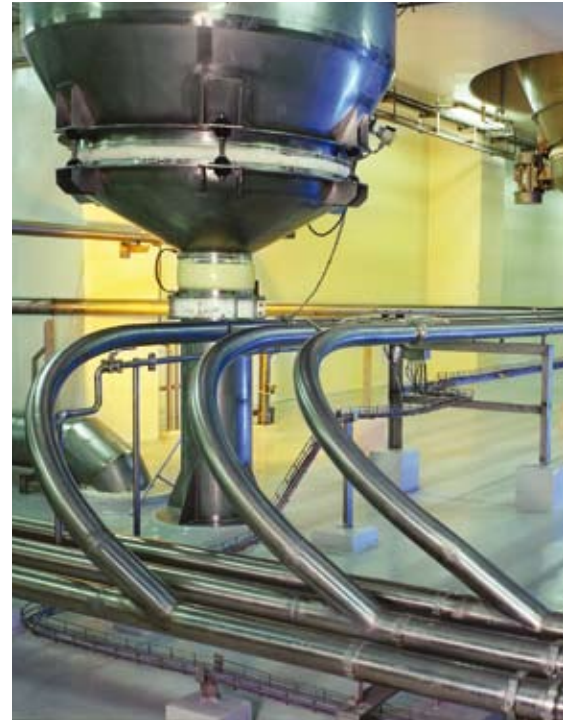
Bottom of powder silos. Pipelines connected for vacuum conveying product to bag filling machines
